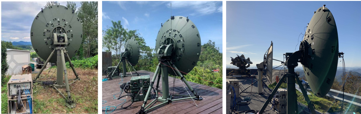
Modular Transportable Transmission System (MTTS)
